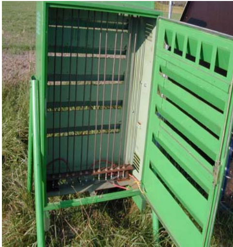
Figure 4.28: The housing of the heating elements
